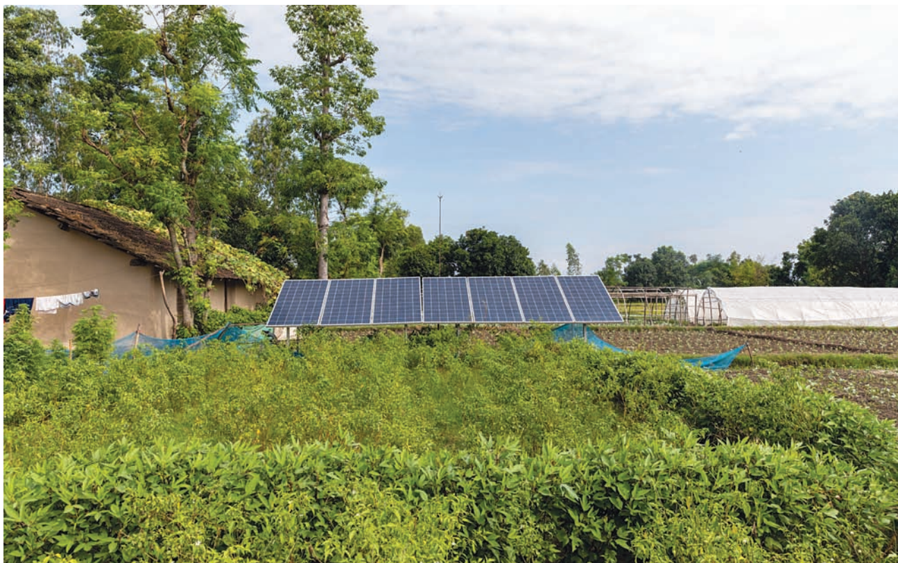
Community Solar Water Lifting Scheme in Bardiya.
